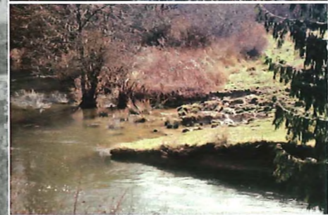
The two images above show bank erosion along the Millstone River at Biggs Road.
