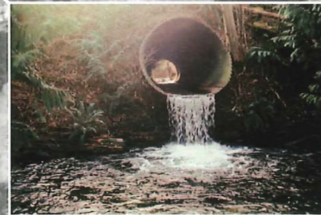
The culvert at McClure Creek and Jingle Pot Road is an obstruction that prevents fish passage as it is perched over one metre above plunge pool.
