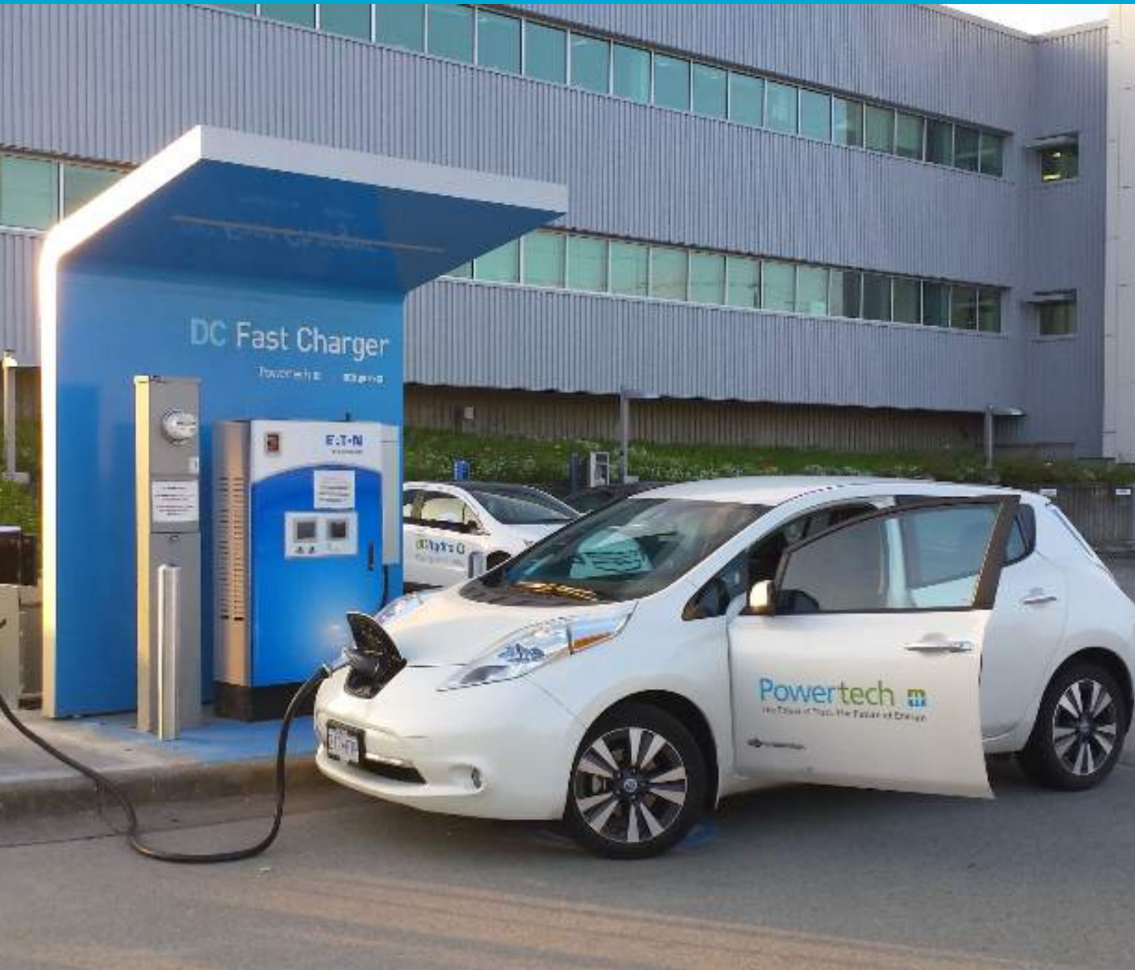
BC Hydro EV Charge Park at Powertech Labs – Multi-DC Fast Charger Station for Advanced Operations Testing
