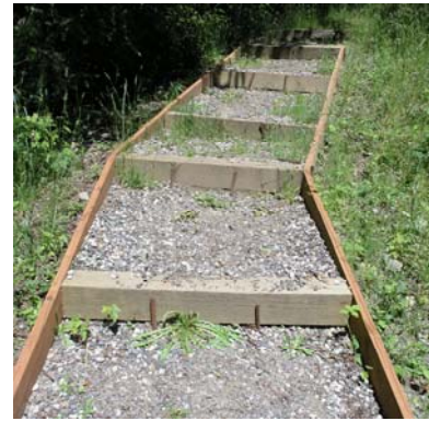
Dirt filled and timber steps like those above have become maintenance concerns and are no longer a park standard.
