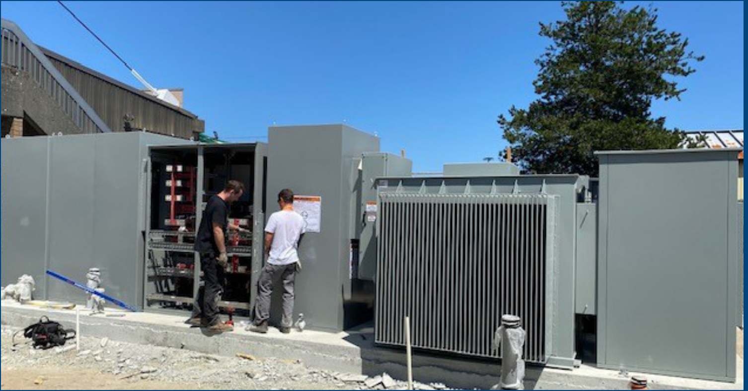
New electrical substation at Beban Park Recreation Facility
