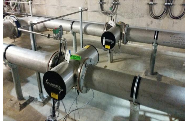
Secondary membranes raw water uv treatment
