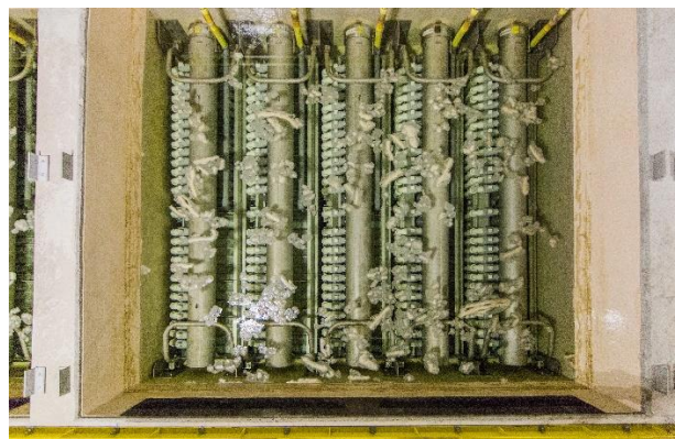
Raw water being filtered in primary membranes
