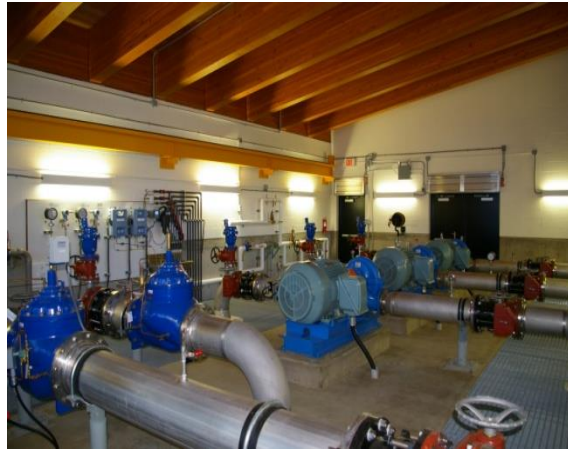
Turbines inside the Energy Recovery Facility
