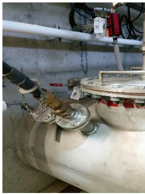
Primary and secondary membrane filtered water being treated at the chlorine injection point
