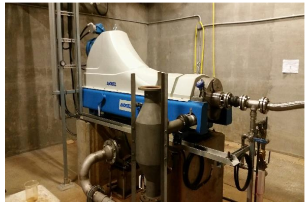
Reject raw water centrifuge
