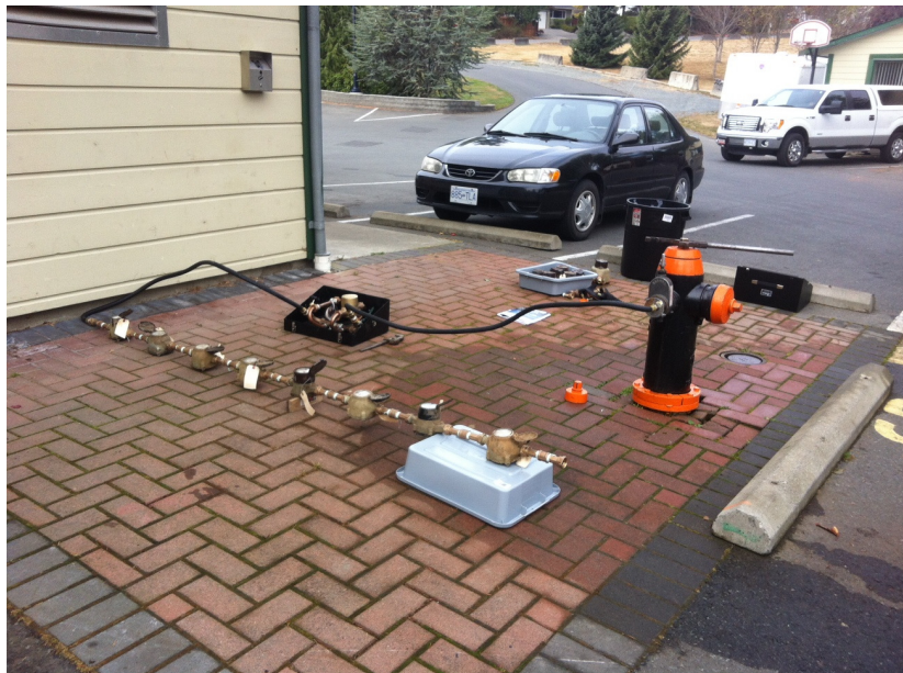
Figure 3-4: Residential Meter Testing
