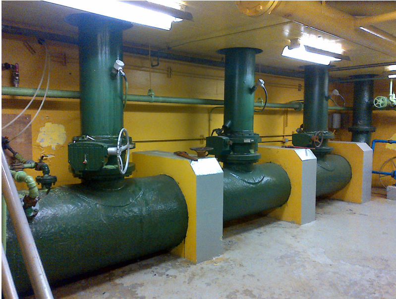
Figure 2-4: Location of Three Source Meters at Water Process Centre
