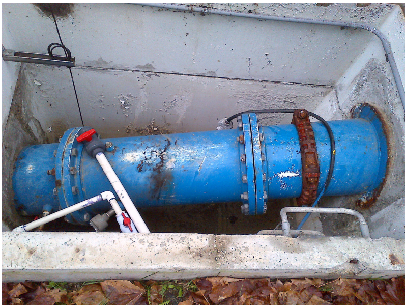
Figure 2-5: One of the Two Source Meters at Reservoir #1
