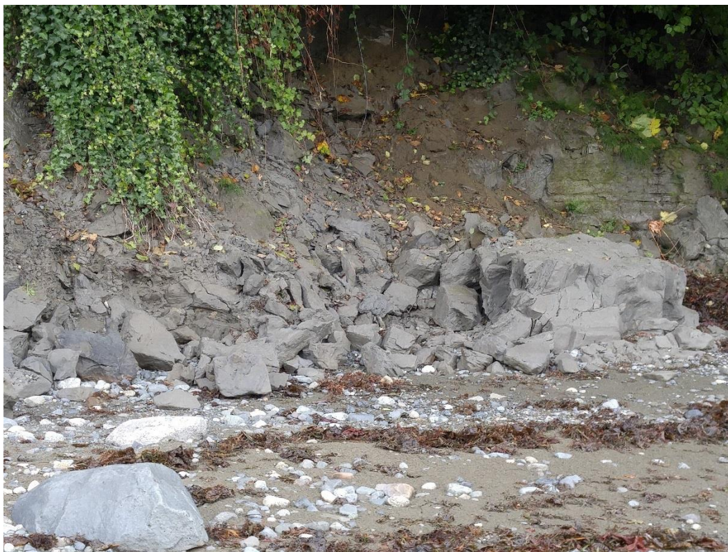
Figure 1-4 Evidence of slope failure; close to Driftwood Place 2017 3
