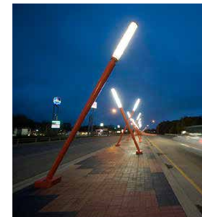
Entry street lighting
