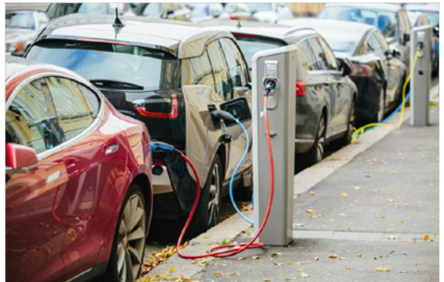
Electric vehicle charging stations
