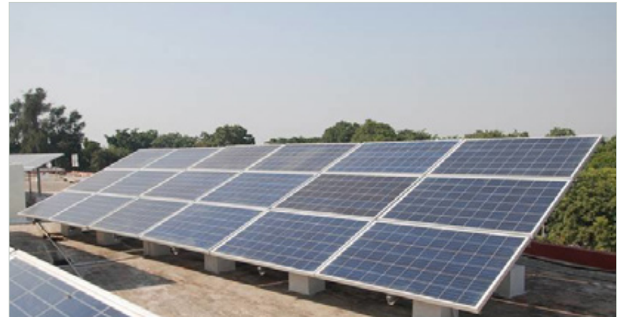
Rooftop PV system
