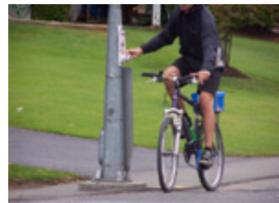
Example of pedestrian push button installations.
